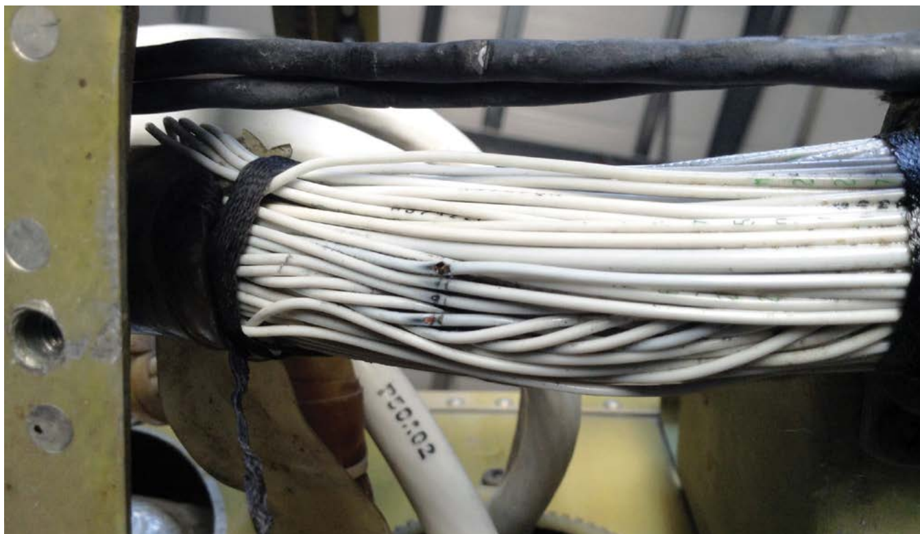
A close-up look at the cause of the perpetual problem – a small black mark on part of a wire bundle.
